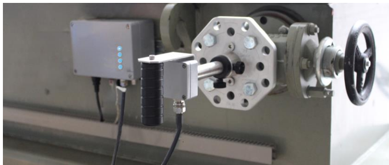
Figure 4 UHF monitoring system installed at a transformer with UHF drain valve sensor at a DN50 gate valve
