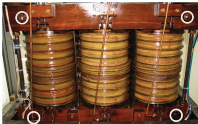
Figure 4. Active part of test transformer. Threaded bolts (see marking) apply horizontal clamping forces to the core sheets.
