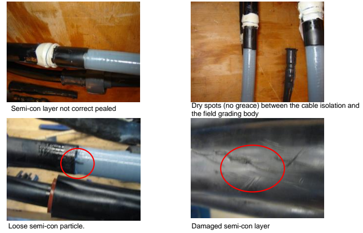
Figure 5. Investigation of the terminations at 0 m location having PD up to 3500 pC at 2 U_0 .
