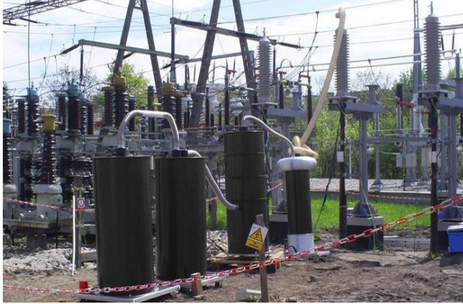
Figure 1. On-site application of a damped AC test system (DAC HV Technology) for a monitored after-laying test with on a 4.5 km long 110 kV power cable
