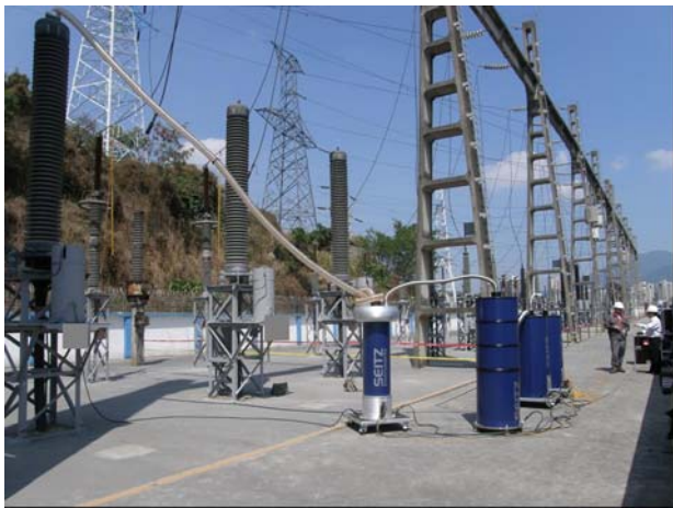
Figure 2 Modern monitored on-site testing and diagnosis with damped AC voltages on a 220 kV cable circuit.
