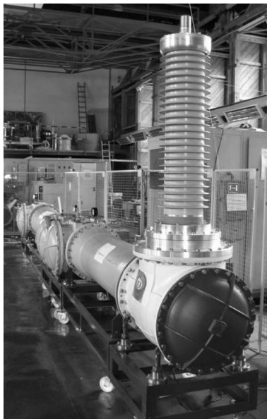
Figure 2: The high voltage test setup in the laboratory of University of Stuttgart: ABB 550 kV GIS type ELK-3 with bushing
