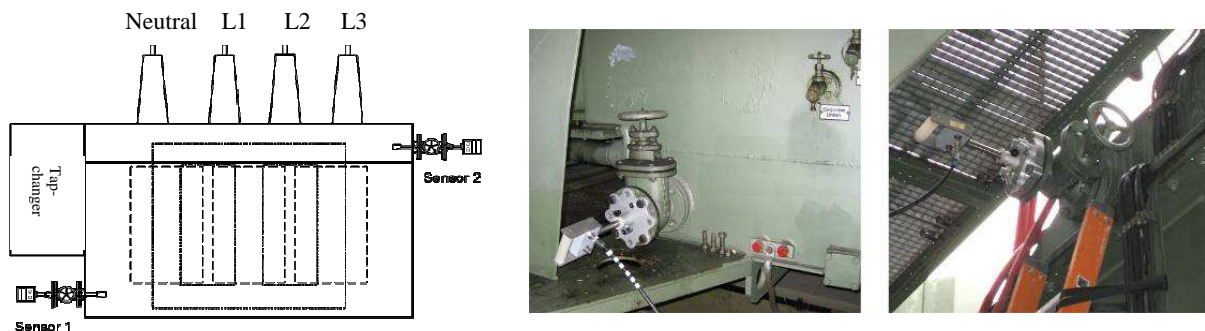
Figure 1: UHF probes installed at a 120 MVA generator step-up transformer
