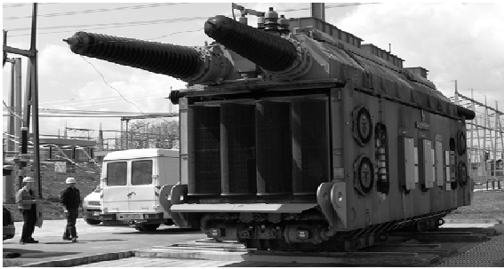
Figure 5: 210 MVA Grid-Coupling Transformer
