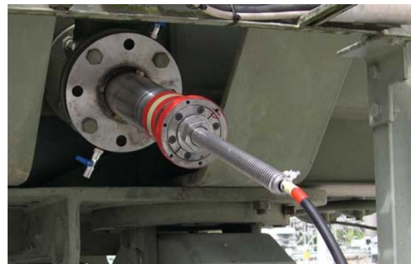
Fig. 11 : The installed disc-shaped UHF-sensor for standardized valves (installed in service)
