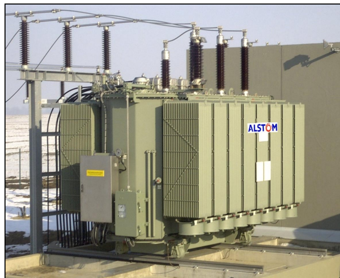
Fig. 5: Hermetically sealed power transformer 80 MVA / 110 kV
