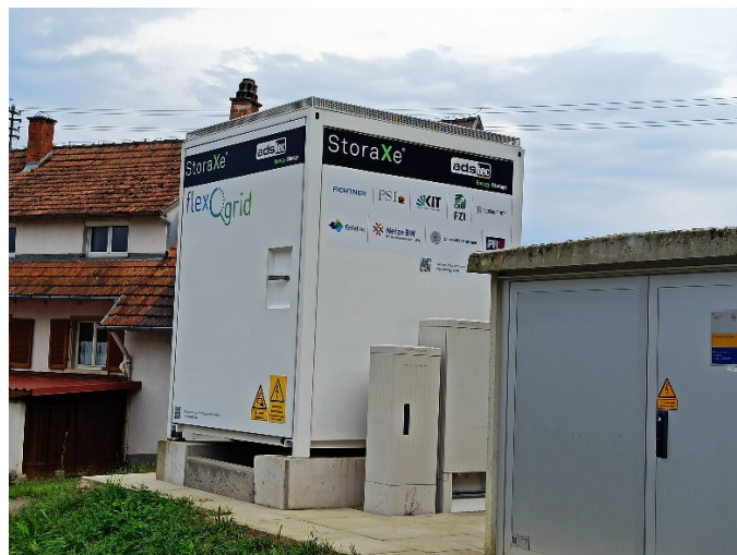
Storage system at field test location
