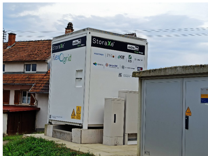
Storage system at field test location
