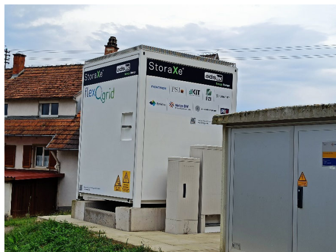
Storage system at field test location
