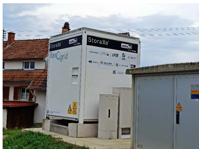
Storage system at field test location
