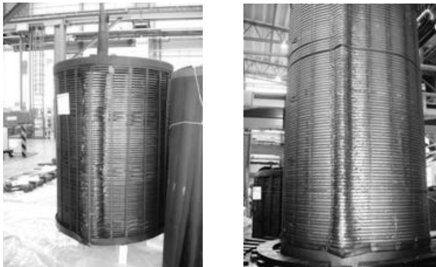
Fig. 2: Kurzschlusschaden (radiale Deformation) an 220/110-kV-Wicklungen Short circuit damage (radial deformation) at 220/110 kV windings
