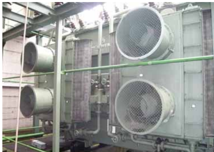
Fig. 2: Maschinentransformator, 125 MVA Generator step-up unit, 125 MVA
